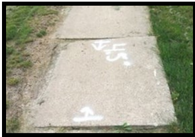
White lines with arrows and a number between them indicates the length of repair, and what panels need replaced.
