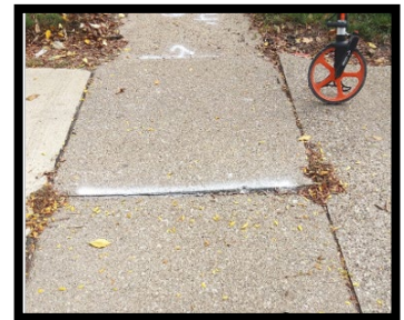
A straight white line with NO arrows indicates that the edge of the panel can be ground down (owner does NOT have to replace entire panel)
